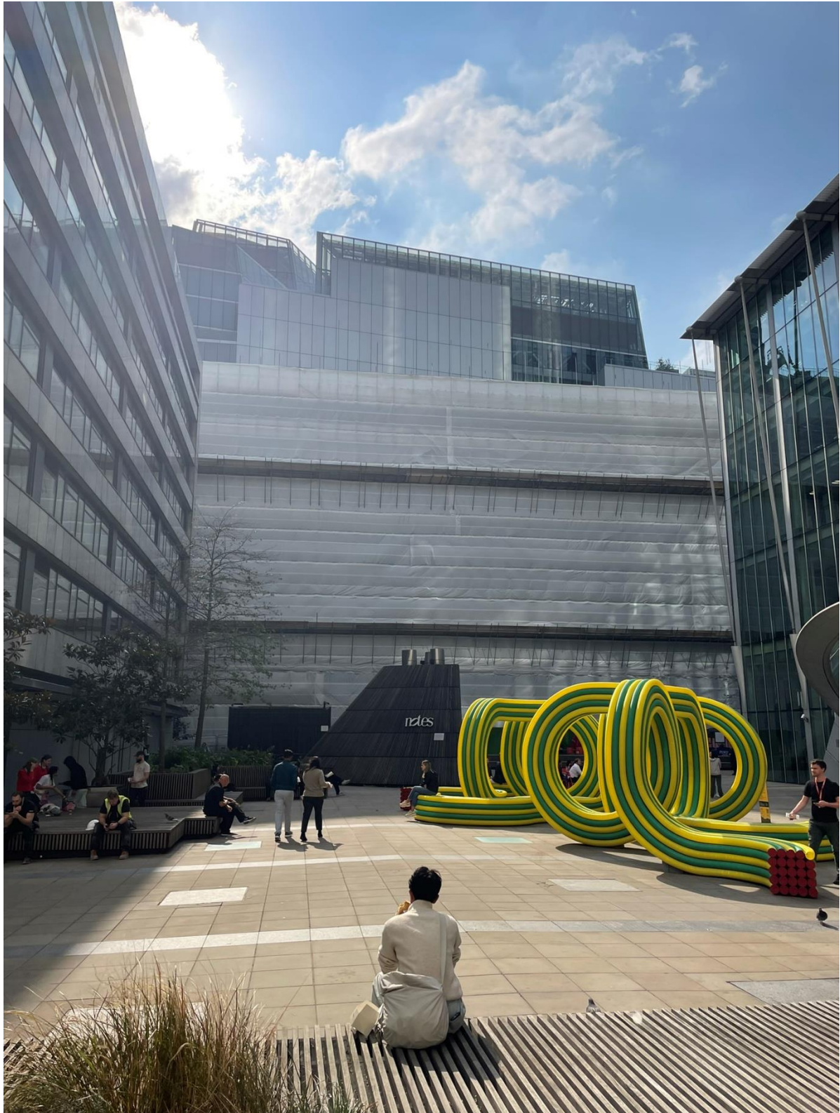
Image 3: North elevation of site under demolition from City Point Plaza (21 Moorfields behind)
